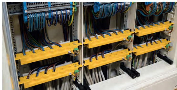
RCMS150 residual current monitors in the installation
